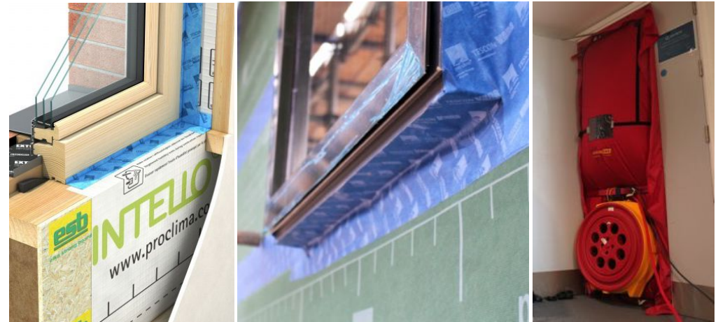
A significant part of reducing energy demand in buildings is minimising heat losses and air leakage and paying attention to detail. Site supervision and empowering construction teams to take responsibility for these performance items is a crucial part of this. The images above show techniques for reducing and testing for air leakage. This can be achieved by using off the shelf products and considering construction sequence from an early stage.
