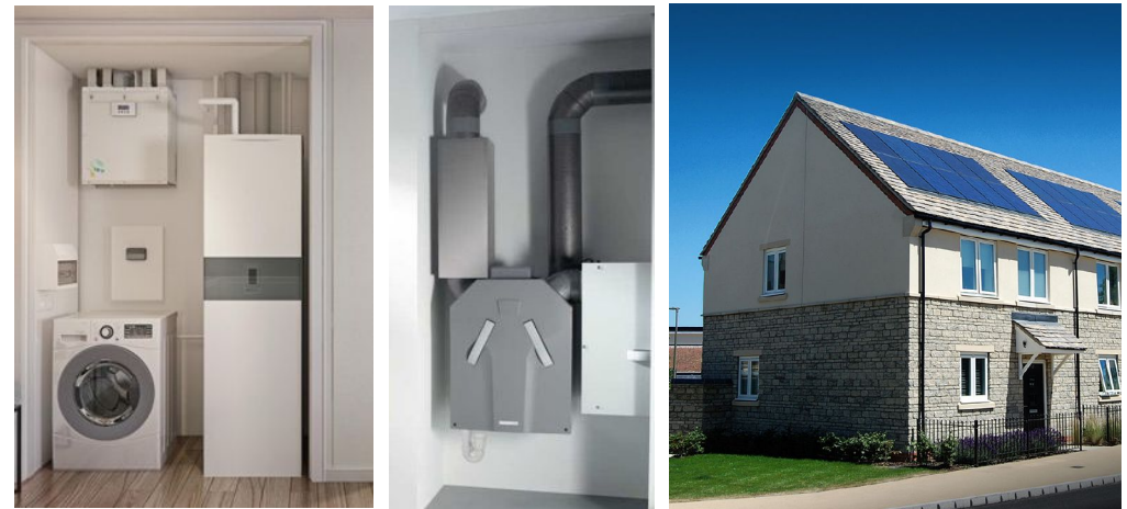
Technology that drives down energy consumption is easily available. Designers and contractors must however allow for these systems early-on in scheme conception and pay close attention to their installation, commissioning and maintenance. Allowing space on floor plans from an early point in design is crucial. The above images show the integration of (from left to right) an individual heat pump, a mechanical ventilation system with heat recovery, and roof mounted photovoltaics.
